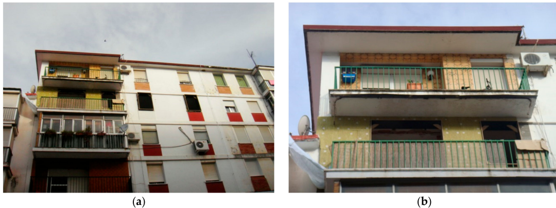
Figure 11. (a) Exterior façade of the dwelling under refurbishment; (b) Balcony façade detail.
