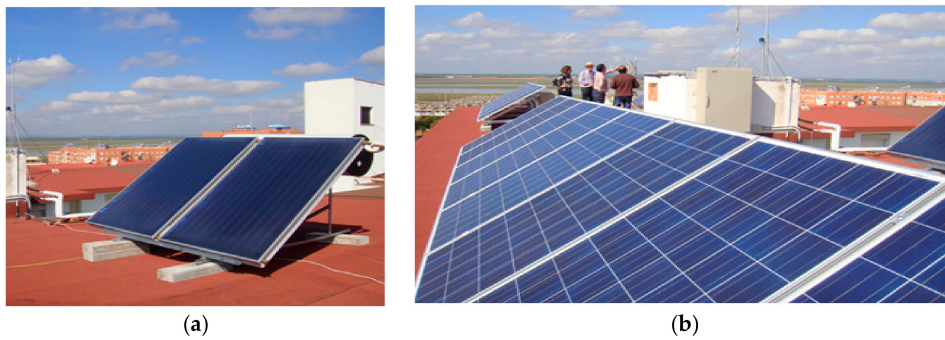
Figure 16. (a) Flat solar thermal collectors; (b) Photovoltaic panel facility.
