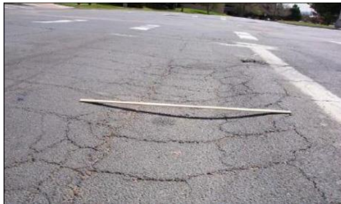
Fig. 2.16. Depression appearing on a pavement surface as a consequence of rutting.
