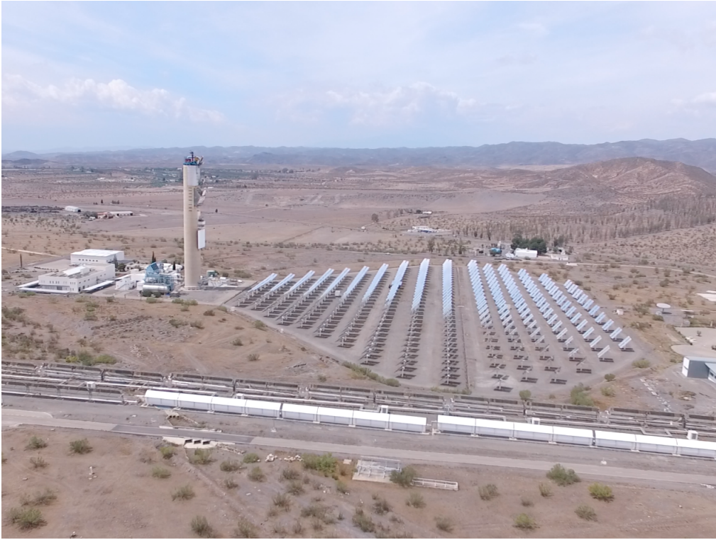
Figure 1: Aerial view of the solar tower power plant at PSA.
