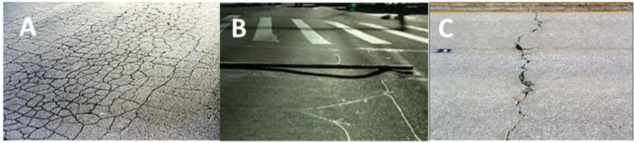
Figure 1.1. Some examples of the different types of distresses: a) fatigue cracking; b) rutting; c) thermal cracking.
