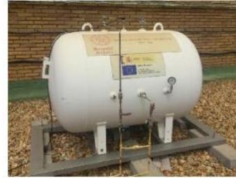
FIGURE 5. Hydrogen high pressure tank.
