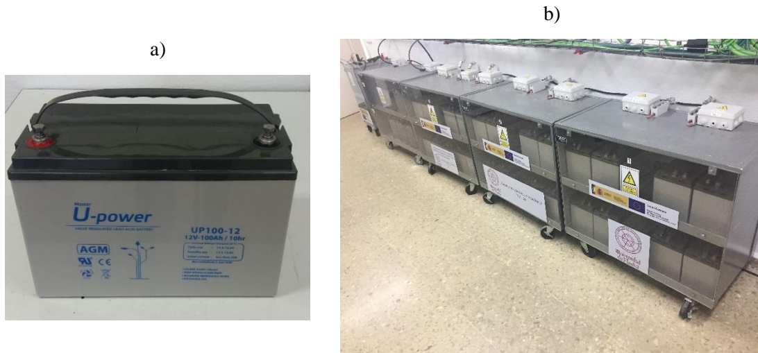
Figure 3.3. Detail of the battery bank. a) UP100-12 single battery. b) Battery bank
