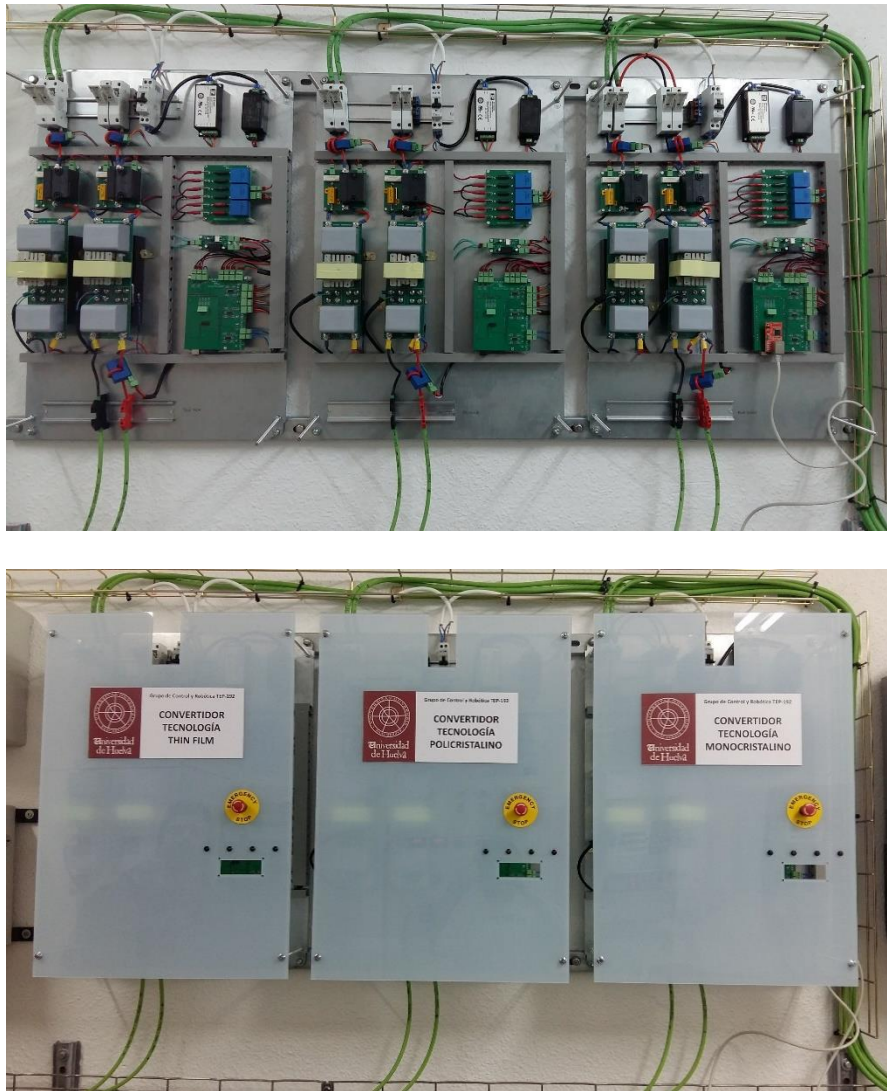
Figure 3.9.- Boost PV-converters prototype and final installation
