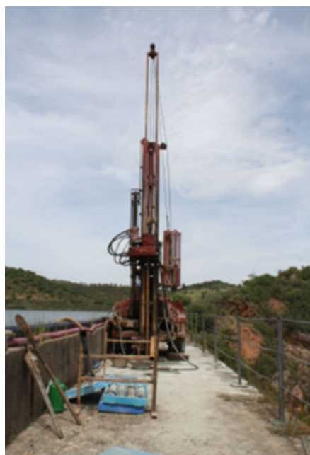
Fig. 9 Detail of drilling machine and core collection at the Alisal-San Miguel Dam
