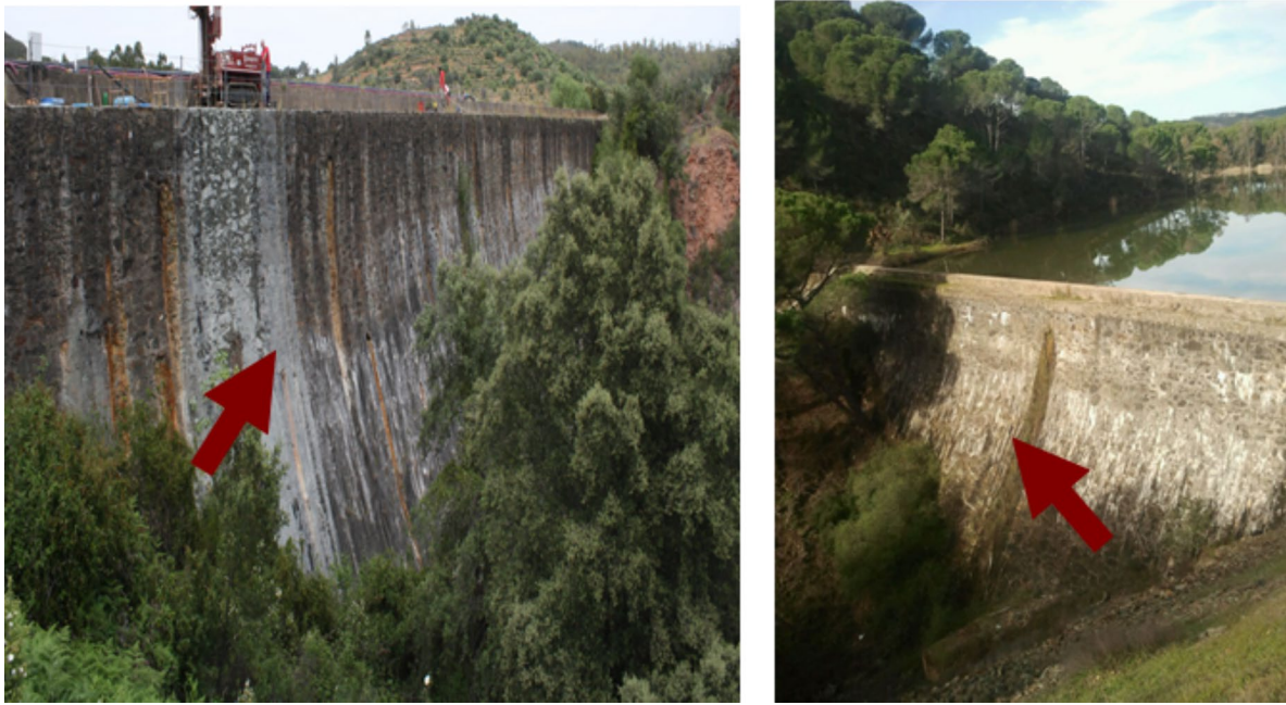
Fig. 14 Location in the areas of anomalies visually detected in the walls of both Dams
