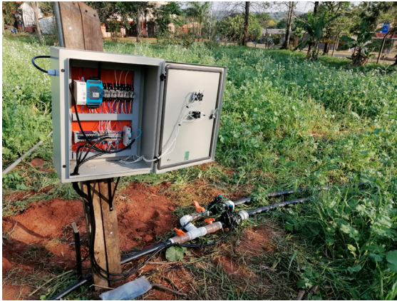
(b) Sensing/actuation node with valves and water meter
