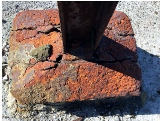
Fig. 8. Concrete support and metal mine beam affected by acidic water.
