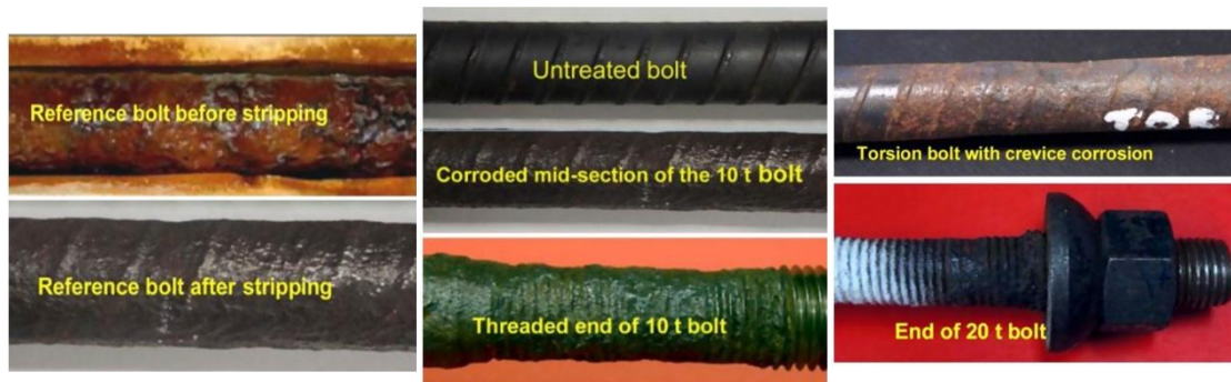
Fig. 7. Photos of parts of various corroded bolt sections compared with uncorroded section [modified from Aziz et al. (2014)]
