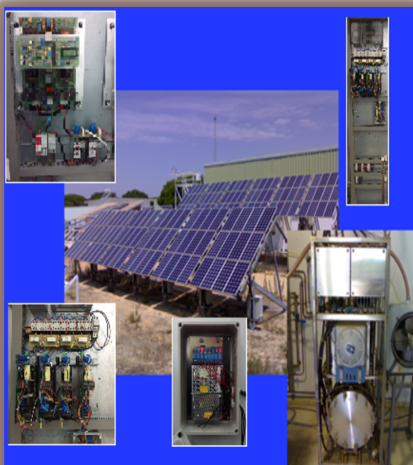
Detail of the power electronics-based installation developed for INTA.
