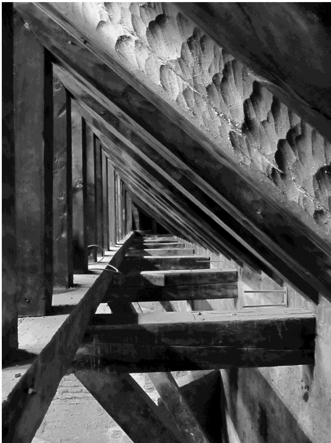
Detail of the roof structure of the nave at Colegial del Salvador church (photo: M. Domínguez Delmás).
