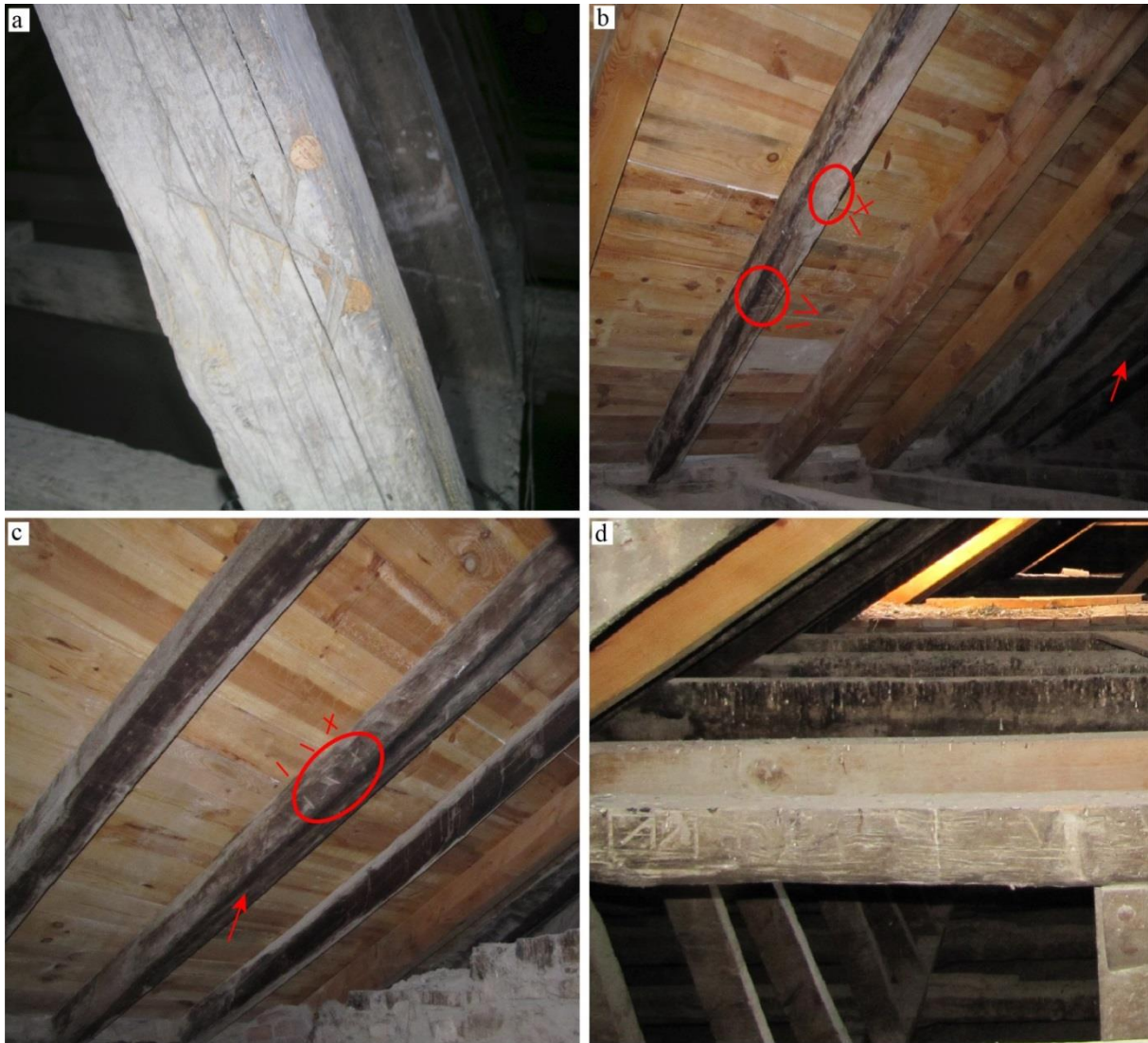
Figure 5. Carpenter marks in timbers from the JCSAC; (a) Mark resembling a five (III) found in the fifth strut from the southern side of the structure; (b) double marking in the 21st rafter of the southern side (the red arrow points at the same rafter pointed at in (c)); (c) mark resembling an eight (IIX) in 25th rafter from the southern side, indicating a consecutive relative position with the mark IV in rafter 21; (d) different annotations in a collar beam that seem to indicate that this timber was reused. Photos: M. Domínguez-Delmás.
