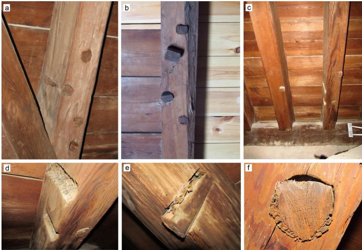
Figure 8. Rafters from the pyramid roof structures of the transepts presenting wooden pegs related to timber rafting (a-d). The pegs are made of deciduous oak ( Quercus subg. quercus ) and are fastened with (or were used to fasten) willow ( Salix sp.) twigs.
