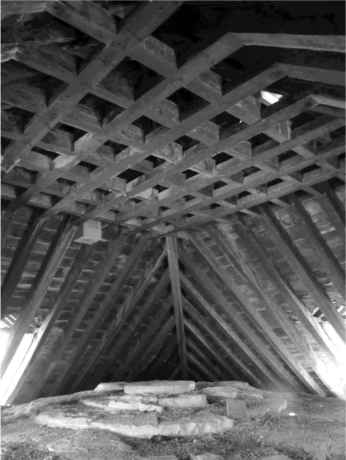
Roof structure of the pyramidal roof above the choir at Jaen Cathedral (photo: M. Domínguez Delmás).
