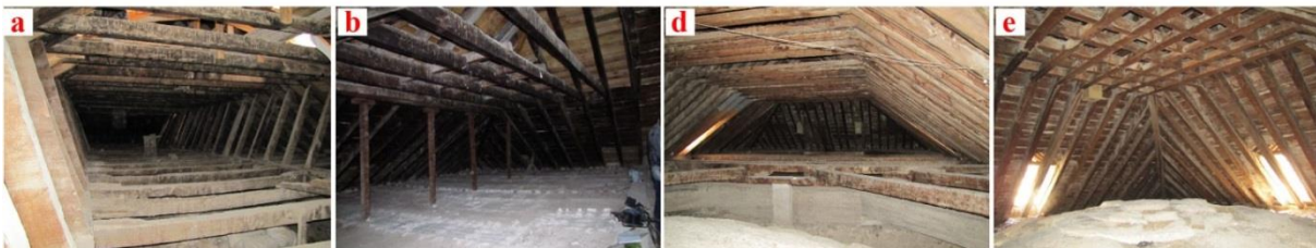
Figure 2. Jaen Cathedral. Top (left to right): facade from the cathedral, and two views from the pyramid above the choir (JCCHO) (Photos: T. Wazny). Researched roof structures: (a) 16th century roof structure above the sacristy (JCSAC), covering the chapter room in the east-end (b), and the antechamber of the sacristy in the west-end (c); (d) 17th century roof structure above the altar (JCALT); (e) 18th century pyramidal roof covering the western dome above the choir (JCCHO). Photos: M. Domínguez-Delmás. Drawing: S. van Daalen and M. Domínguez-Delmás.
